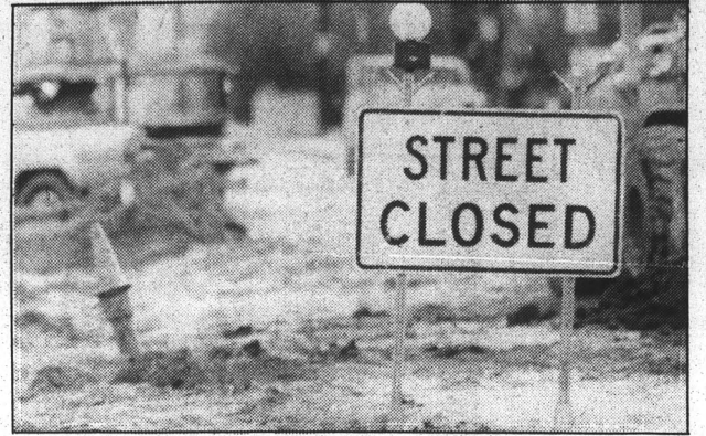
Irwin Daugherty/State Press Road construction has forced the temporary closure of McAllister Avenue, making both vehicle and pedestrian traffic hectic for dormitory residents.
