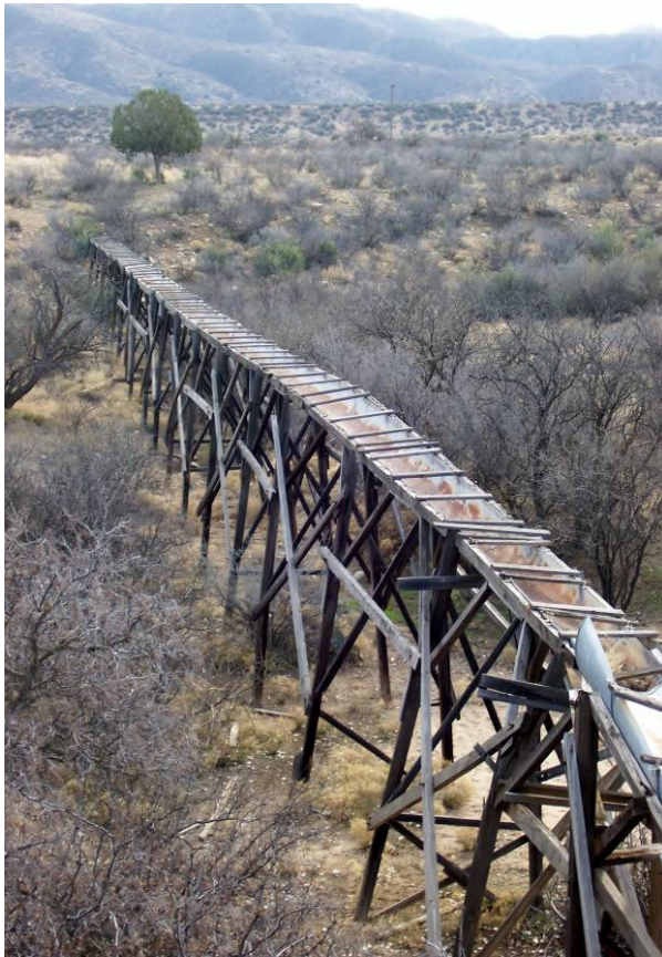
Figure 7 – An unused aqueduct, the Leppe Wash flume, is located on the historic TK Bar Ranch along the Hassayampa River near Kirkland, Arizona.
