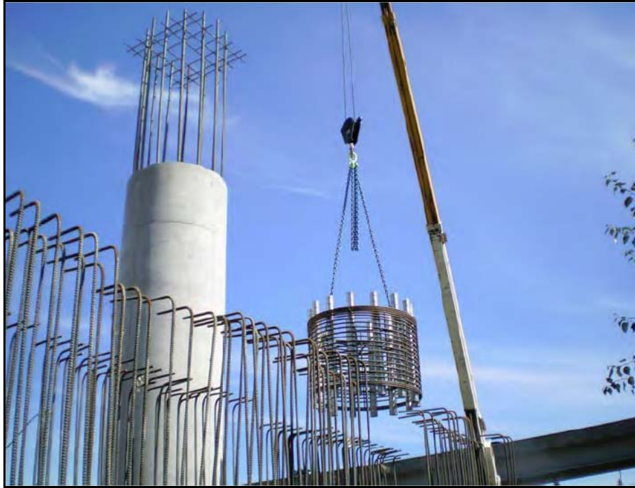
Figure 33. Template for Aligning Column Bars and Bent Cap Connection Ducts. (Pang et al. 2008.)
