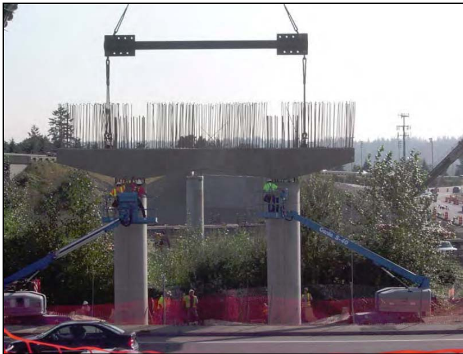
Figure 34. Precast Bent Cap in Place on SR 520 / SR 202 Interchange Flyover Ramp. (Pang et al. 2008.)
