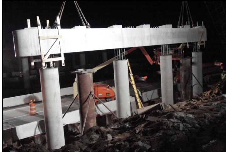
Figure 13. Precast Bent Cap Being Lowered into Position on Parkview Avenue Bridge. (Cooper 2009, courtesy of MDOT.)
