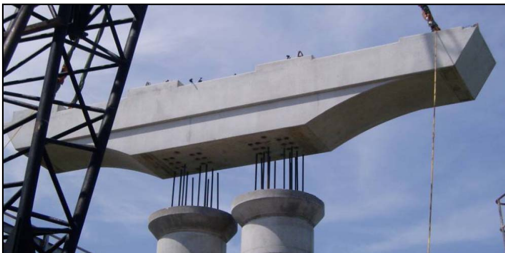
Figure 24. Precast Cap Beam Being Lowered into Position on Lake Belton Bridge. (FHWA 2009.)
