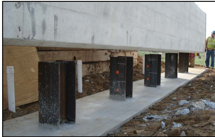
Figure 11. Precast Pile Cap Being Lowered into Position on Parkview Avenue Bridge. (Photo Courtesy of MDOT.)
