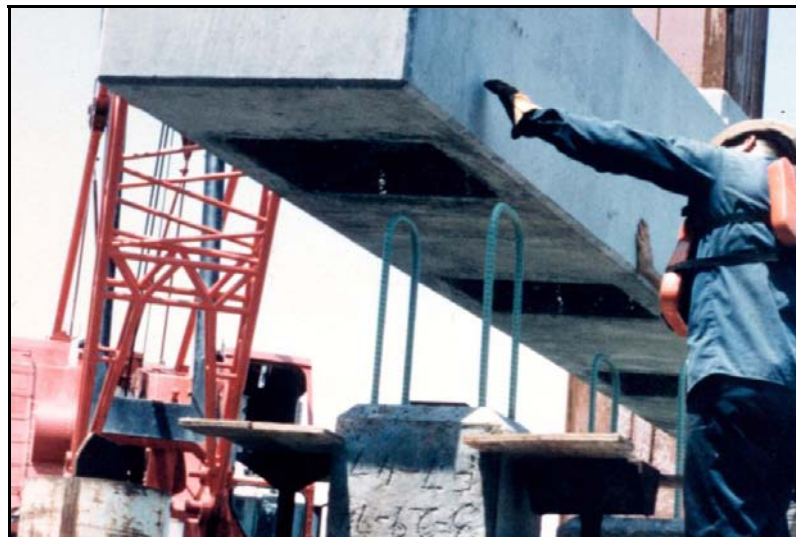
Figure 17. Precast Cap on Red Fish Bay and Morris and Cummings Cut Bridge. (Wolf 2005.)
