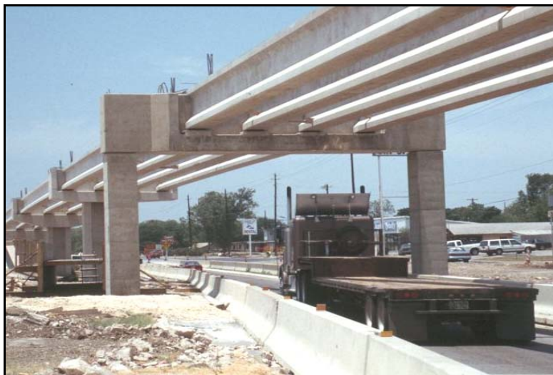
Figure 21. Precast Superstructure Beams Resting on Precast Bent Cap on Ramp E-3. (Marin 2008.)
