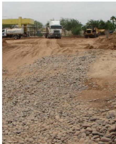
Poorly maintained gravel pad
