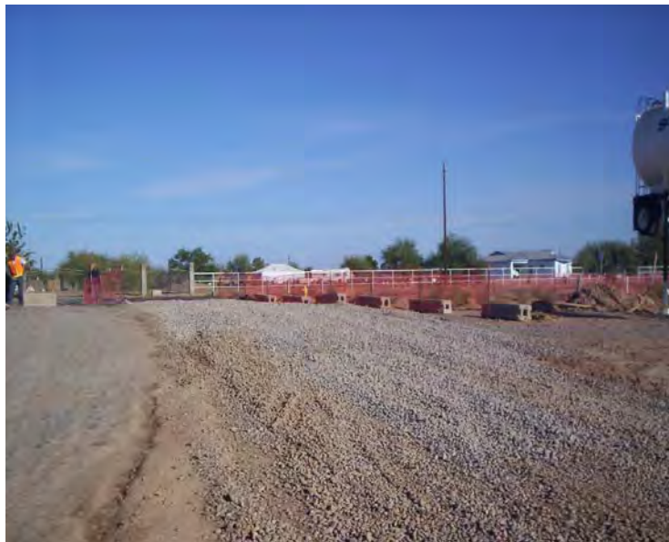
Gravel pad at permitted area entrance/exit
