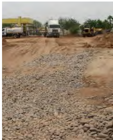
Poorly maintained gravel pad
