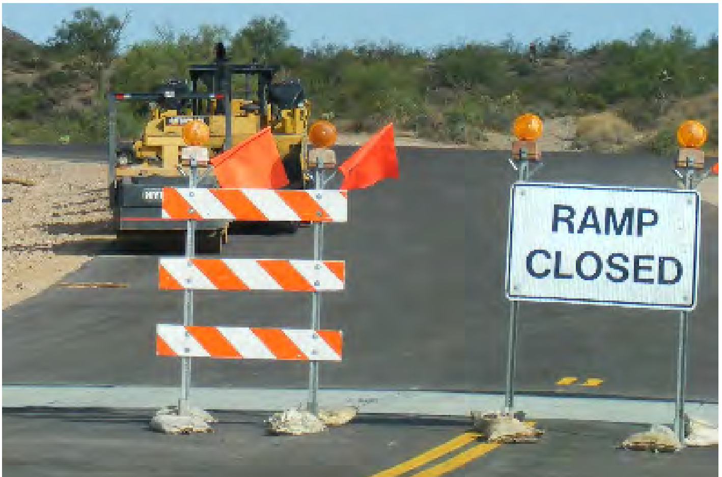
Signage restricting access to paved area
