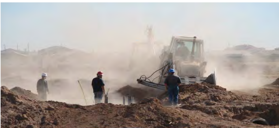
This activity resulted in a notice of violation being issued to a block permit holder
