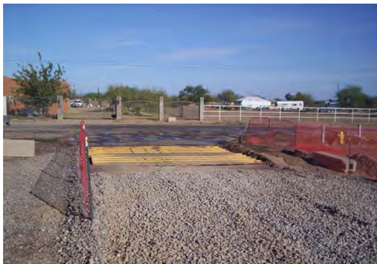
Here a grizzly has been added to the gravel pad as an extra control measure
