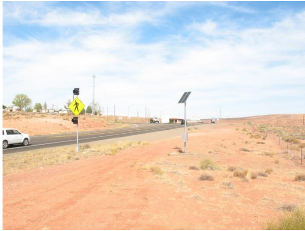
Pedestrian Warning Signage and Beacons
