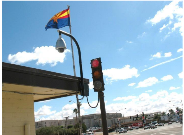
Lane Control Signal Downstream of Scale
