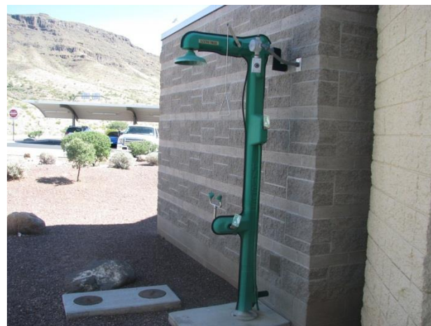
Emergency Shower and Eye Wash Facility
