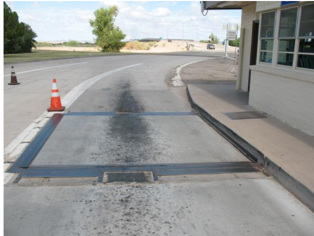
Inbound Static Scale West of Admin Building
