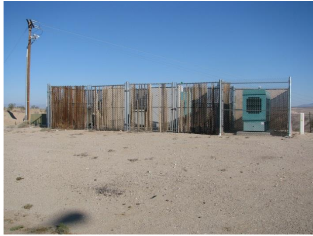
Emergency Power Generator for the POE
