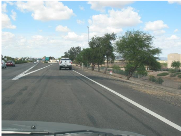
Skid Marks at I-8 WB POE Off-ramp
