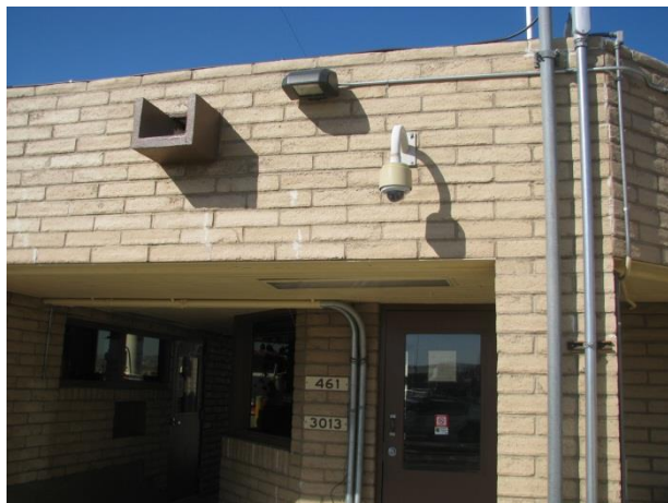
Admin Building Security Camera and Lighting
