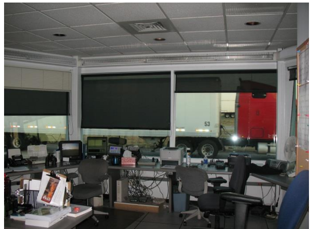
Main Control Room
