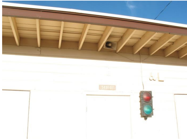
Green/Red Control Signal and Loudspeaker
