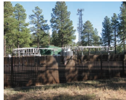
Kachina Village Utilities (top); APS substation and telecommunications tower (above).
