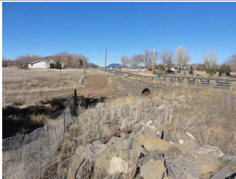
West side of the Koch Field Road bridge south of Kavanaugh / Anaya Road
