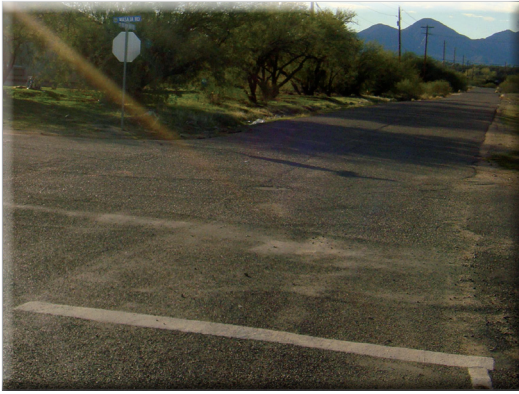
Pavement condition on Wassaja Road at Heque Da Trail
