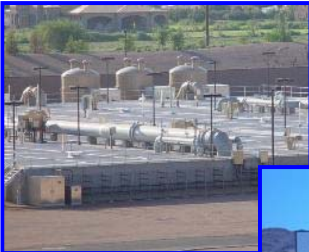
Greenfield Water Reclamation Facility
