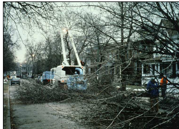
Workers remove trees infested with Asian Longhorned Beetle, chip downed trees in place, and burn the chips.
