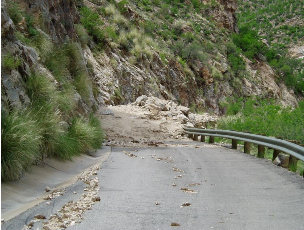
Figure 11. The road to Stop 9. Several debris flows crossed this section of road.
