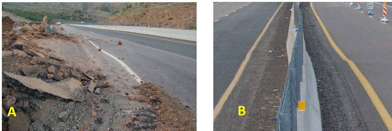
Figure 3 A. Close-up of the lower part of the landslide buckling the highway. B. The landslide displaced the road and divider about 1 foot to the east. Both views looking north. Photos taken on 23 March 2008 by B.F. Gootee.
