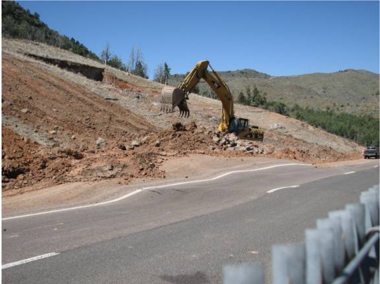
Figure 4 The Easter weekend landslide pushed up the highway, deforming both south- and northbound lanes. The southbound lanes (shown here) buckled approximately 3 feet high and 50 feet along the length of the highway. View is to northwest. Photo taken on 23 March 2008 by M. Diaz.
