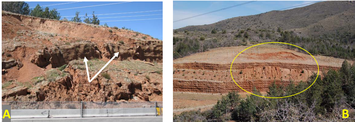
Figure 2. Slope failures that occurred during winter 2007-2008 near mile marker 224. A. The southern-most landslide on the west side of the highway; note the broken shotcrete (white arrows). The metal fence in the foreground is the median of the highway; the Jersey barriers behind the fence are on the shoulder of the southbound lane, separating the highway from debris. B. Slope failure (inside yellow ellipse) in material from an older landslide on the east side of SR-87. Scarps are present above the highest tier of soil nail walls; material is moving down slope over both walls. Photos taken on 23 March 2008 (A) and 25 March 2008 (B) by M. Diaz.
