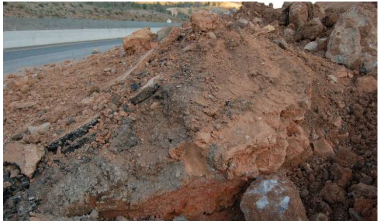
Figure 6 Portion of the Easter weekend landslide that damaged the highway. Note pavement, gray artificial fill under the pavement, and red, clay-rich, moist sediment under the fill. Photo by B.F. Gootee, 23 March 2008.
