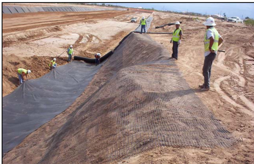
Fig. 16 – Earth fissure mitigation effort on roadway in Pinal County, AZ (photo by Ken Euge)
