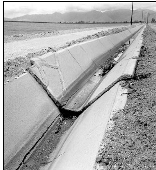
Fig. 2 - Irrigation canal in west Maricopa County broken and offset by subsidence (photo by L. Fellows)
