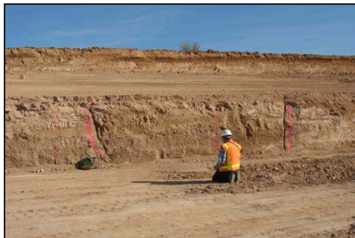
Fig. 11 – Earth fissure cracks below Loop 202 Freeway construction in Mesa, AZ (photo by Ray Harris)
