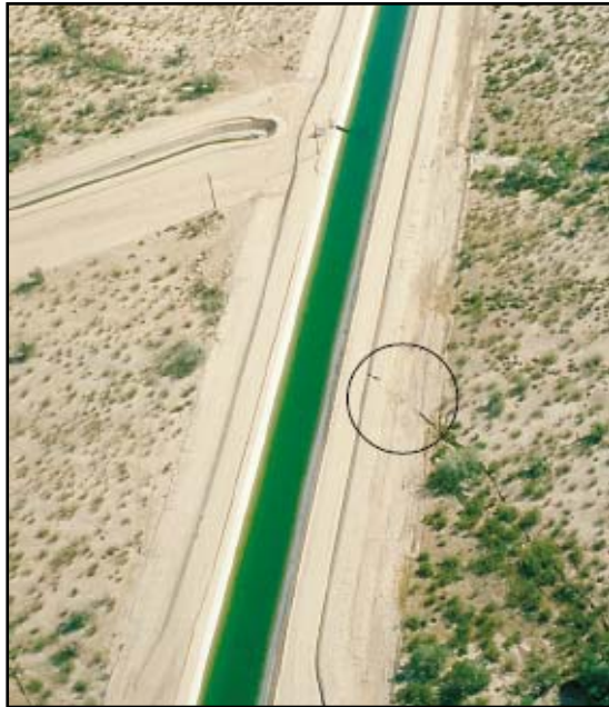
Fig. 10 - Central Main Lateral Canal of the CAP crossing the Picacho earth fissure (fissure shown as a dark line) (photo by Michael Carpenter)
