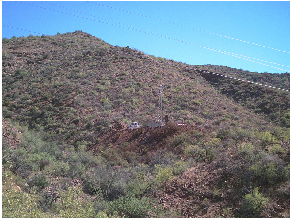
Air drill, set up on TG-1, located on top of the trace of the Potter Ranch Fault zone, just uphill from the Greenlee County Road on the Potter Ranch property.
