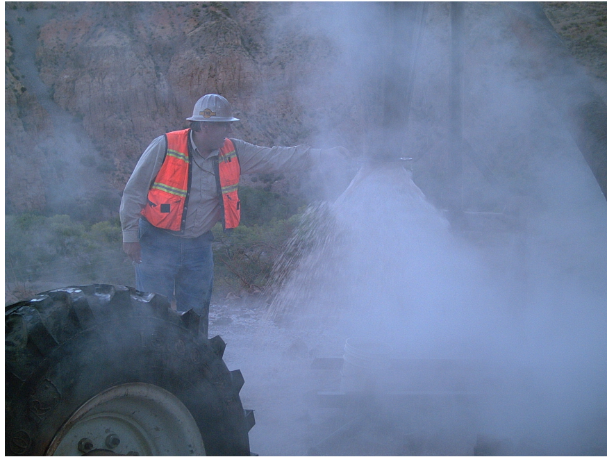
Taking blooie line temperatures on TG-1 at about 400 feet in depth, during air drilling phase.
