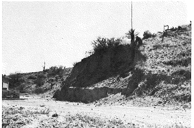
Photo 4. Failure of a cut-back slope. During the summer rains of 1973, many tons of material were released into the backyard. Rilling and piping erosion is now causing further instability.
