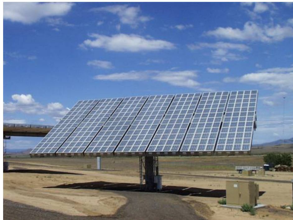
Arizona Public Service photo: Prescott 35 kW, dual axis tracking system.
