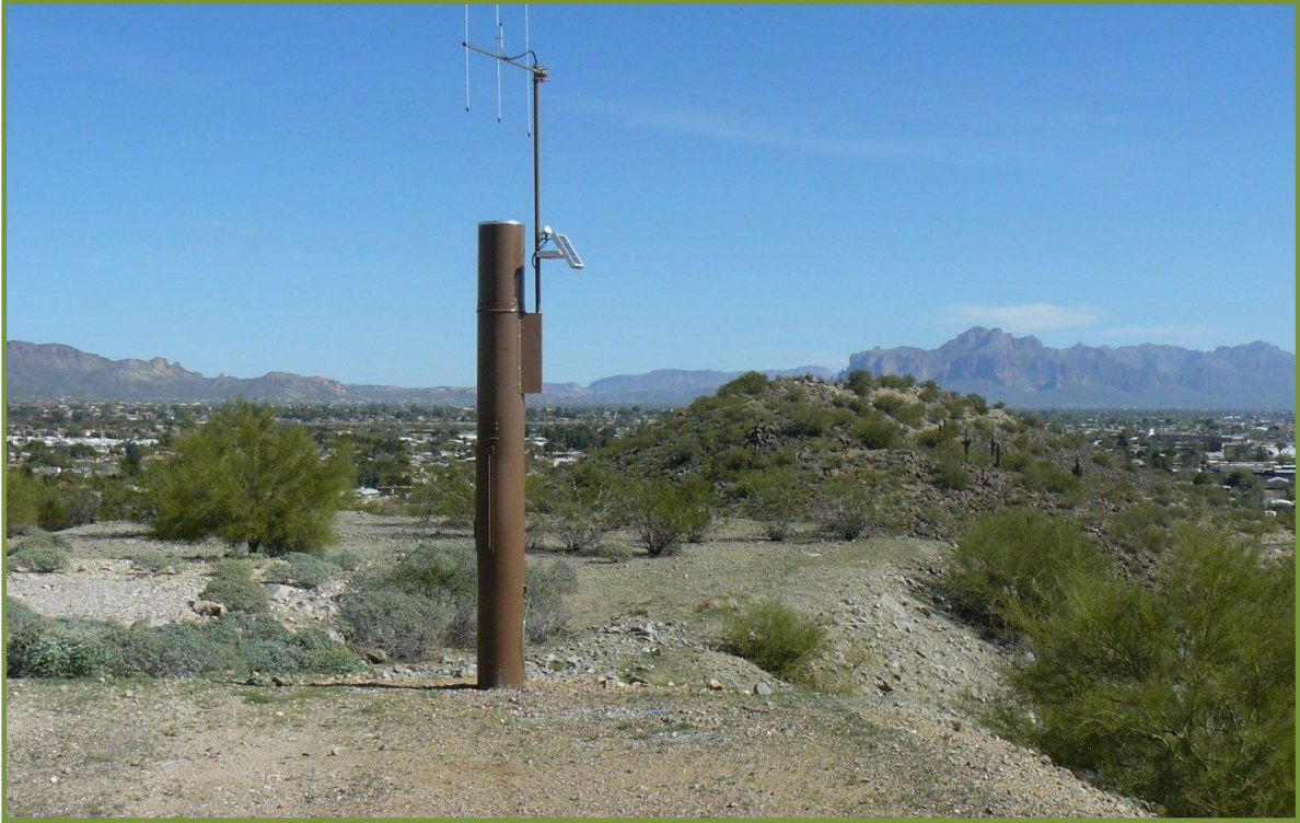
Main St. @ Hawes Rd. Rain Gage, Station 50347, Installed 01/19/2017
