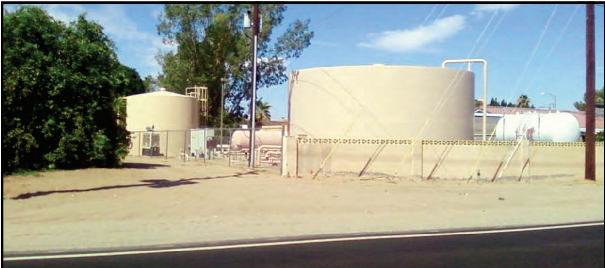
A Small Community Water System in Unincorporated Yuma County
