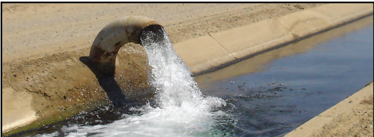
Drainage Well Discharging into a Drain
