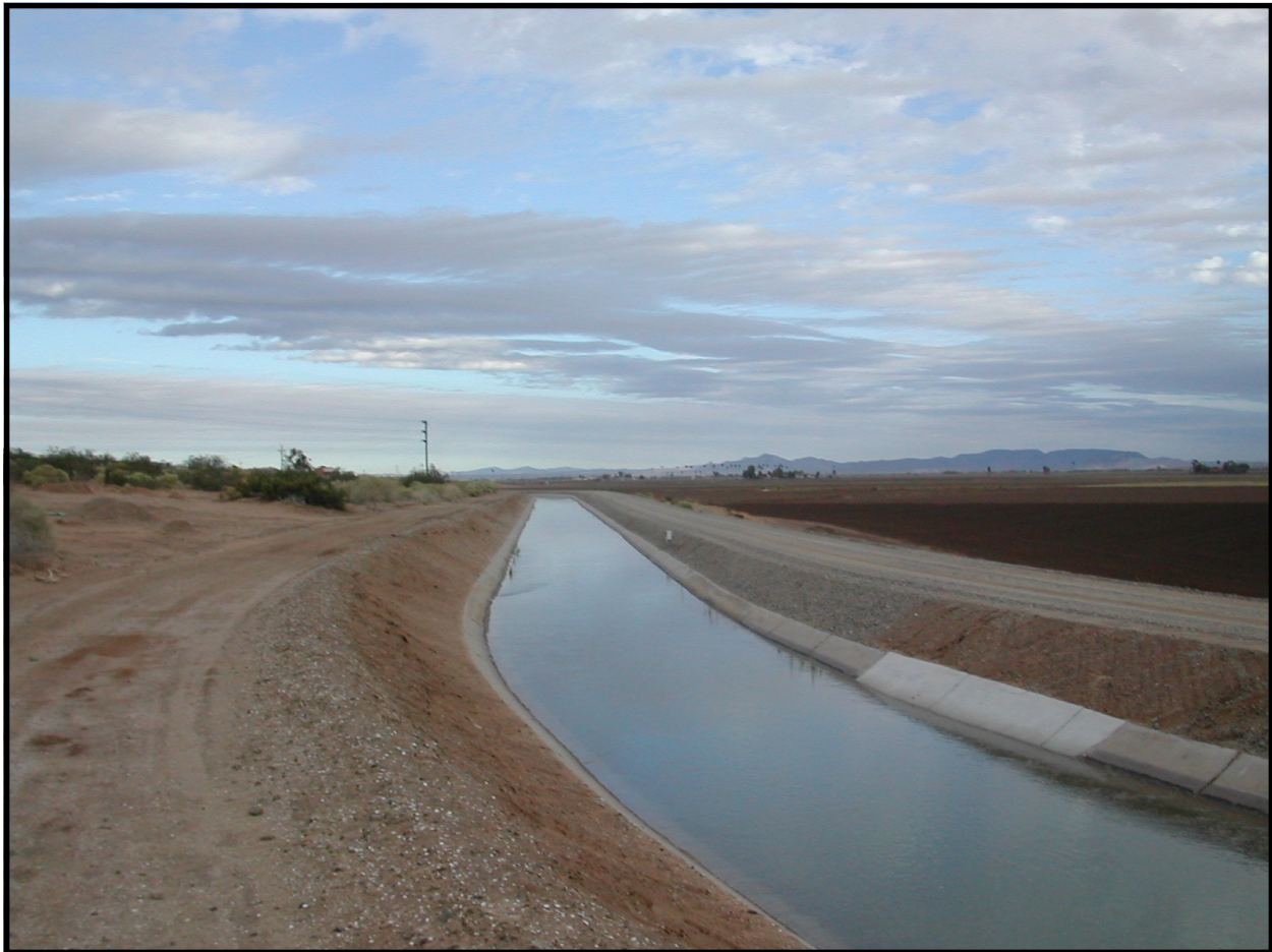
Figure 19: South Gila Valley Main Canal
