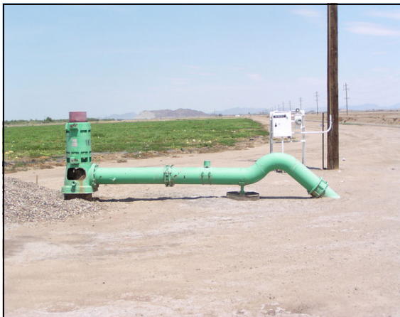
Figure 17: Typical Drainage Well 4
