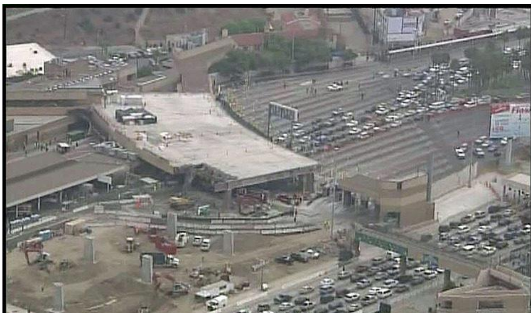
Figure 10: Collapse of San Ysidro Port of Entry Roof
