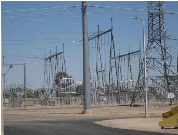
Electrical Transmission Center
