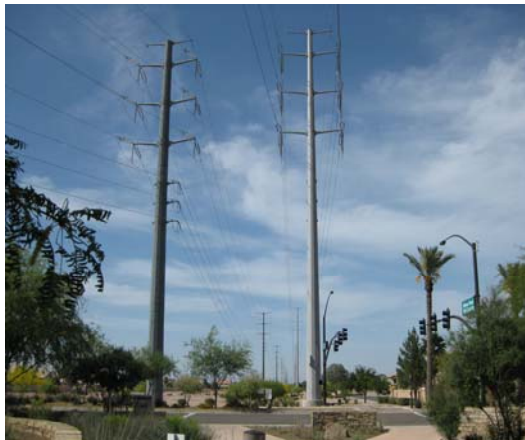
Major Power Transmission Corridor
