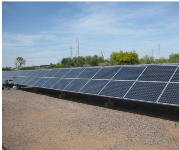
Gilbert APS Solar Power Plant
