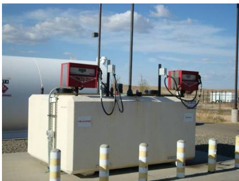
Fuel Farm Pump Station
