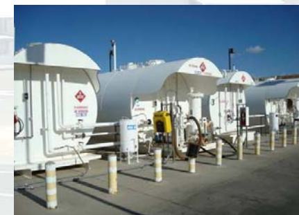
Fuel Farm Storage Tanks
