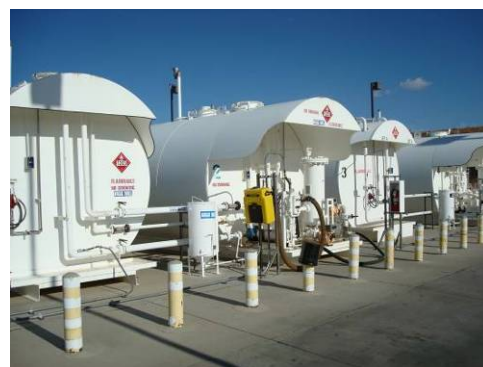
Fuel Farm Storage Tanks
