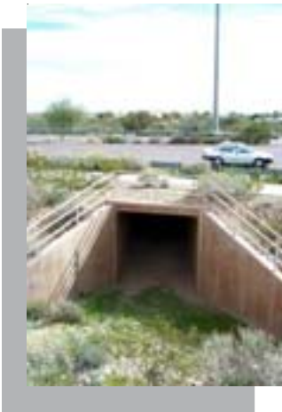
Several drainage structures provide trail crossings under Shea Boulevard
