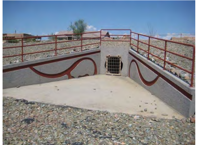
The outlet for the new Pinnacle Peak Channel—a key drainage facility in northern Peoria.
