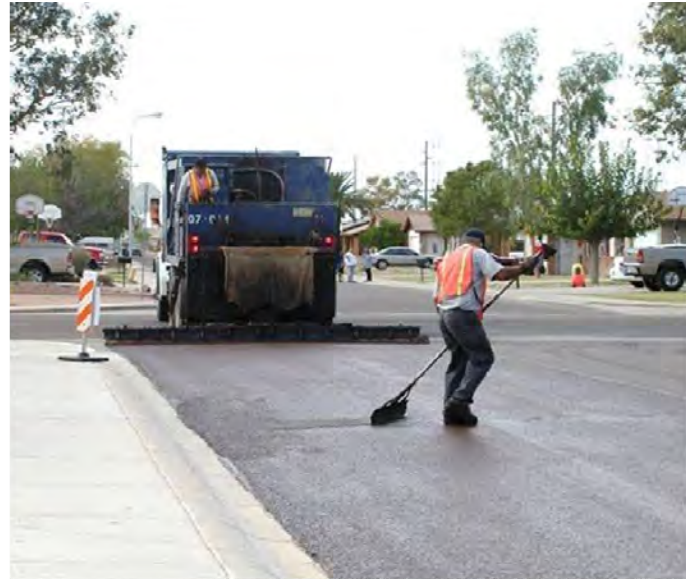
A streets crew performs maintenance work on a residential street in Peoria. The operating and maintenance costs of new infrastructure is a key factor in capital planning.
