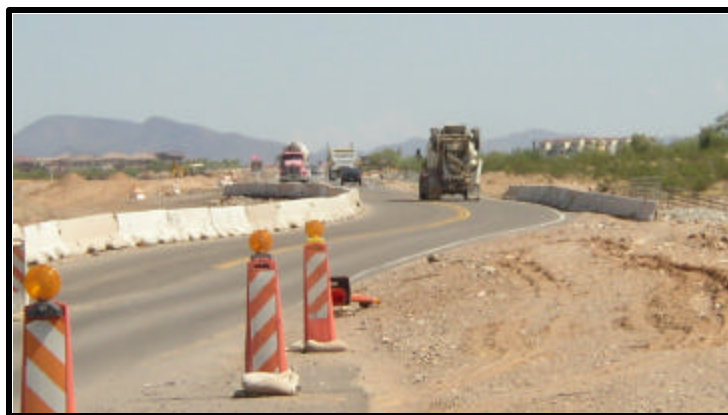
Construction is underway along 99 th Avenue to build improved roadways which will help traffic flow in the Lake Pleasant area.
