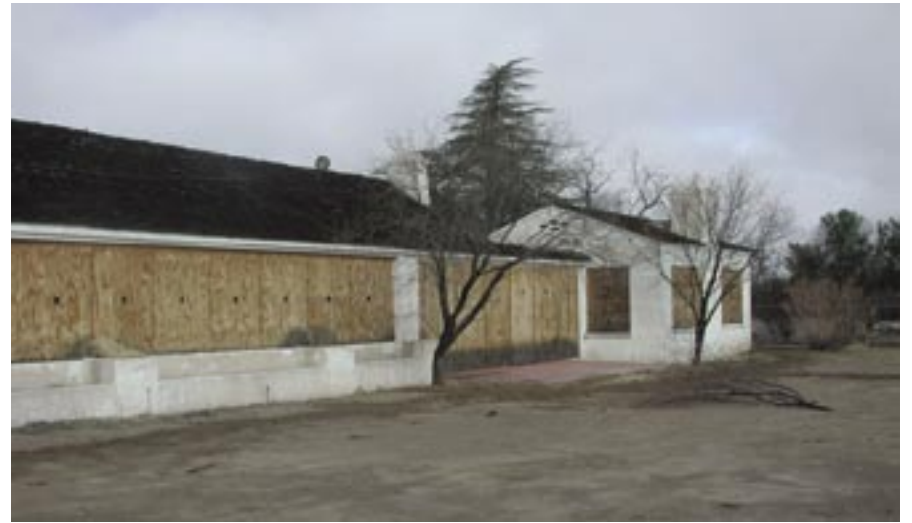
View of east elevation from the southeast Photo courtesy of Poster Frost Associates, 2004
