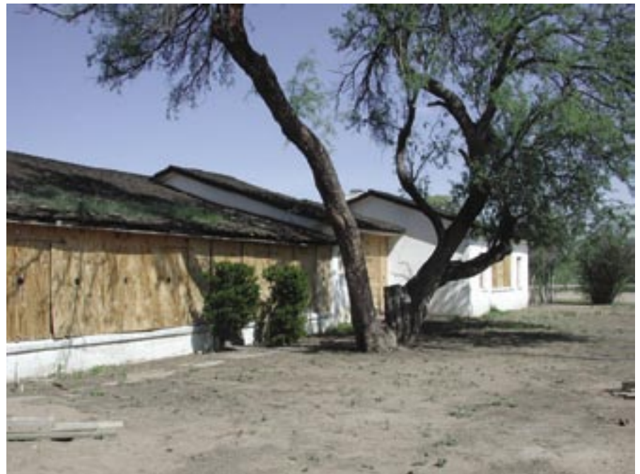
View of east elevation from the northeast Photo courtesy of Poster Frost Associates, 2004
