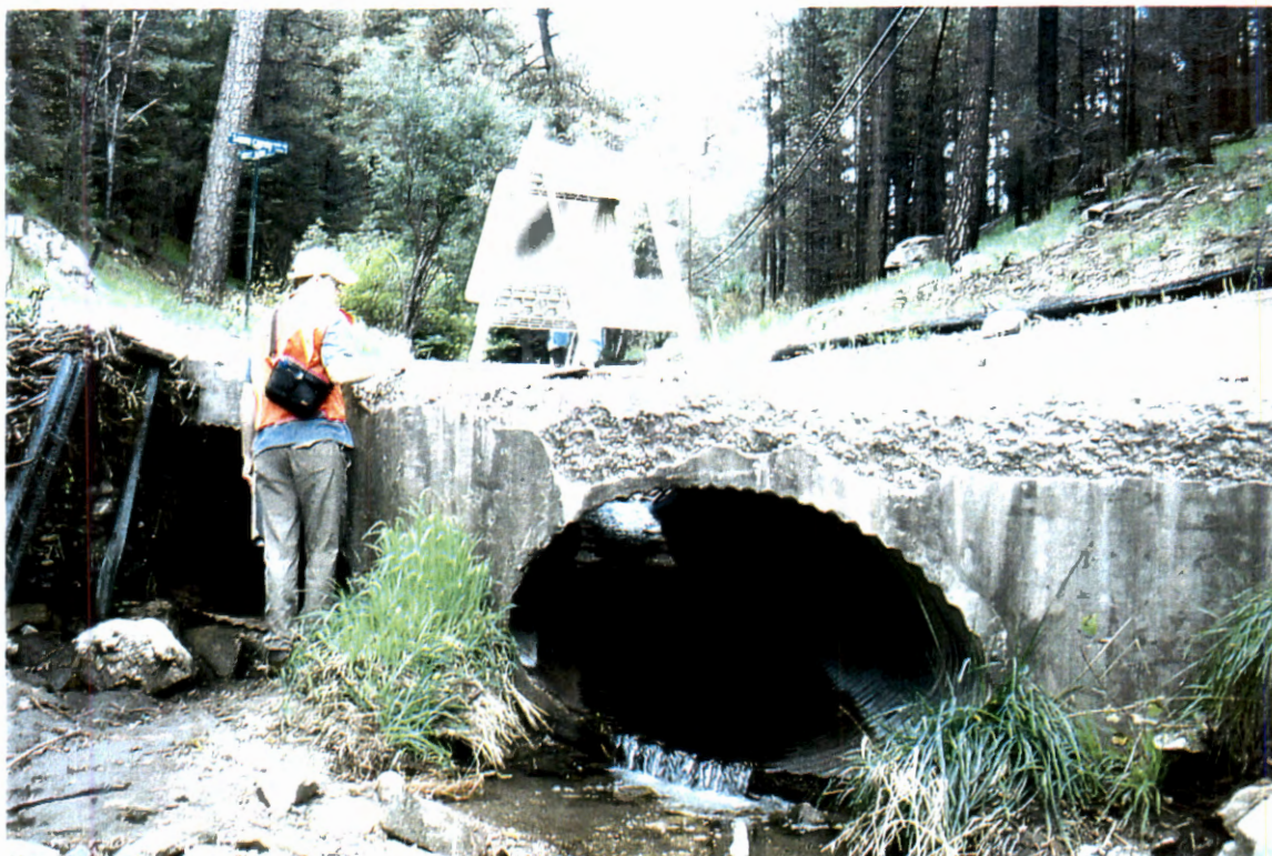
Picture 31. Downstream of East Sabino Road culvert looking upstream at twin ellipse culverts (# 2).
