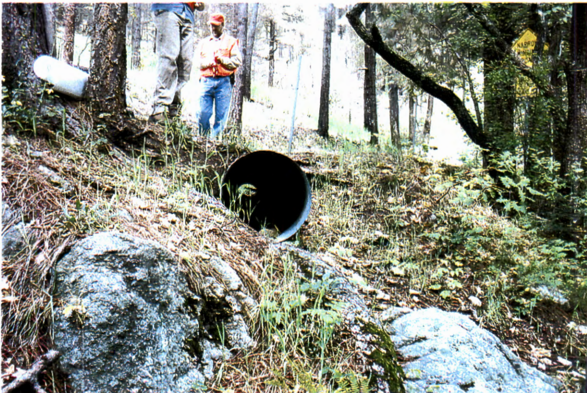
Picture 8. Right side of channel looking upstream at 24" CMP under Sabino Canyon Road.
