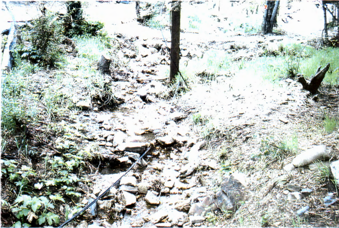
Picture 75. Centerline of driveway culvert (#11) looking upstream at crushed culvert.
