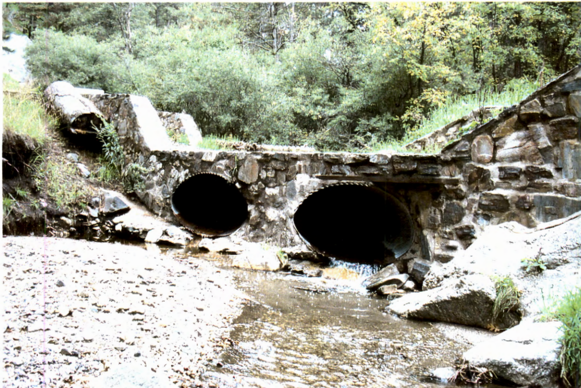
Picture 12. Downstream of parking lot entrance looking upstream at twin ellipse CMP culverts (# 1).
