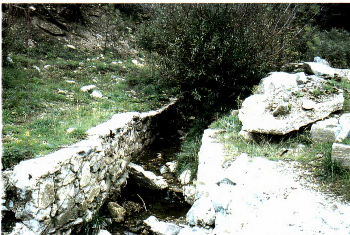
Picture 66. At Sabino Canyon Road looking upstream at channel with retaining walls.
