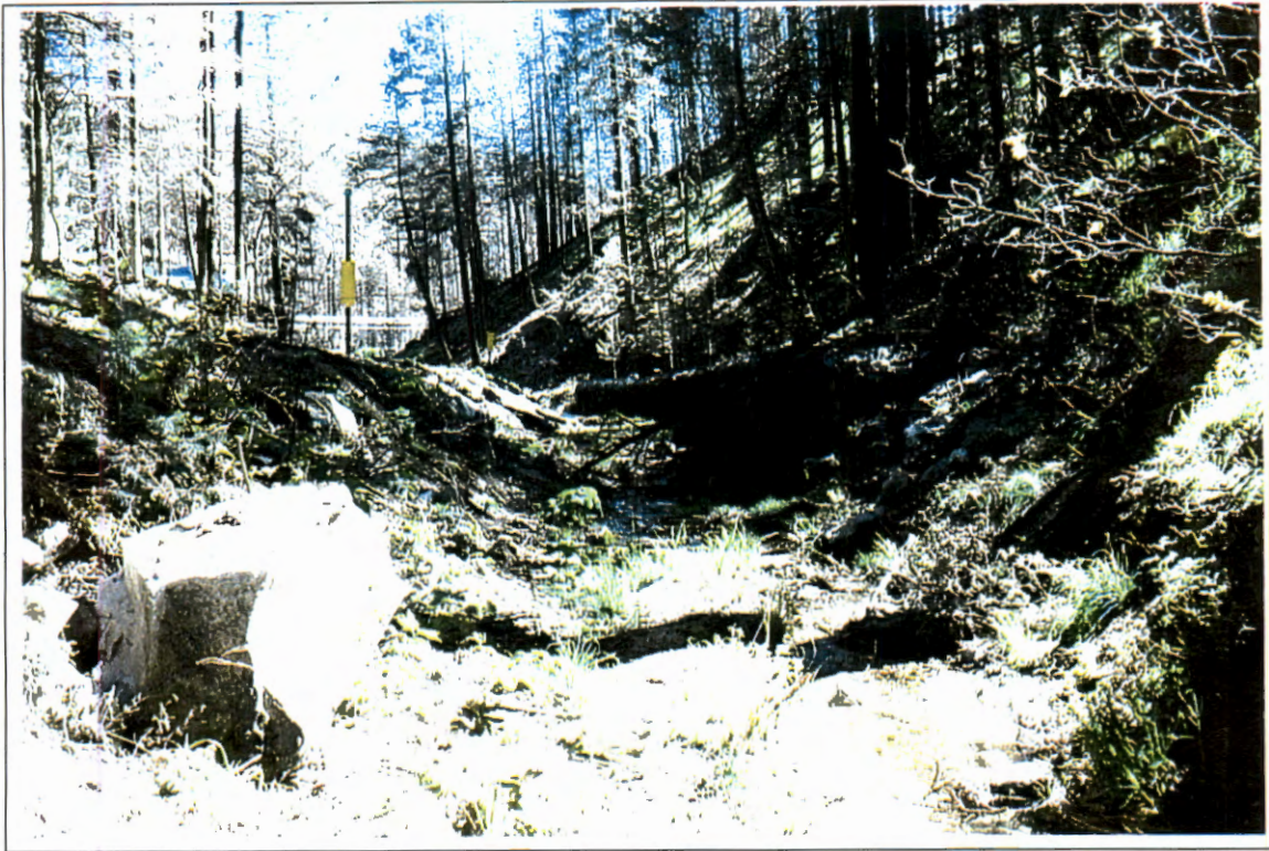
PHOTOGRAPH 128 – 150 feet downstream of driveway culvert along Turkey Run Road (#20) looking downstream. This is an example of high erosion potential.
