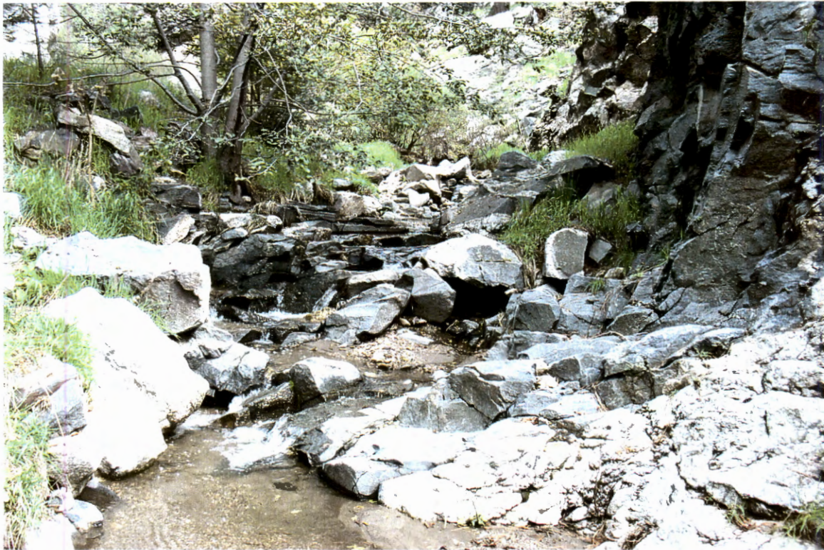
Picture 23. Centerline of channel (100' downstream of panel point) looking upstream at channel constriction and roughness change.
