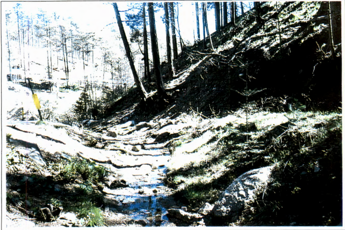
PHOTOGRAPH 130 – 350 feet downstream of driveway culvert along Turkey Run Road (#20) looking downstream. Notice the failing embankment along the right side of the stream.
