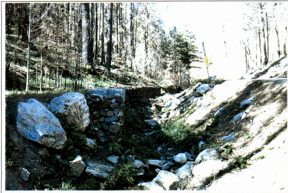
PHOTOGRAPH 129 – 350 feet downstream of driveway culvert along Turkey Run Road (#20) looking upstream. Notice the gabion baskets used to prevent erosion of the stream.
