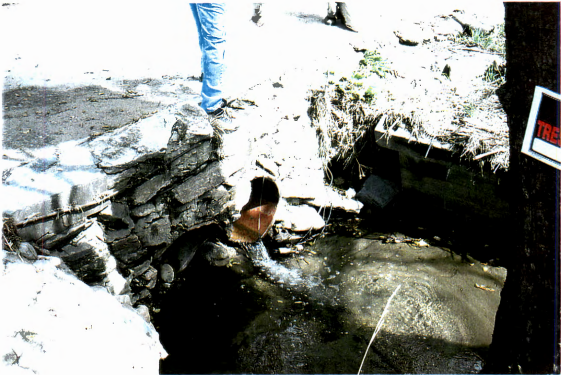
Picture 49. Downstream of driveway culvert at right bank looking upstream at 2-18" clay pipes in concrete (# 5).
