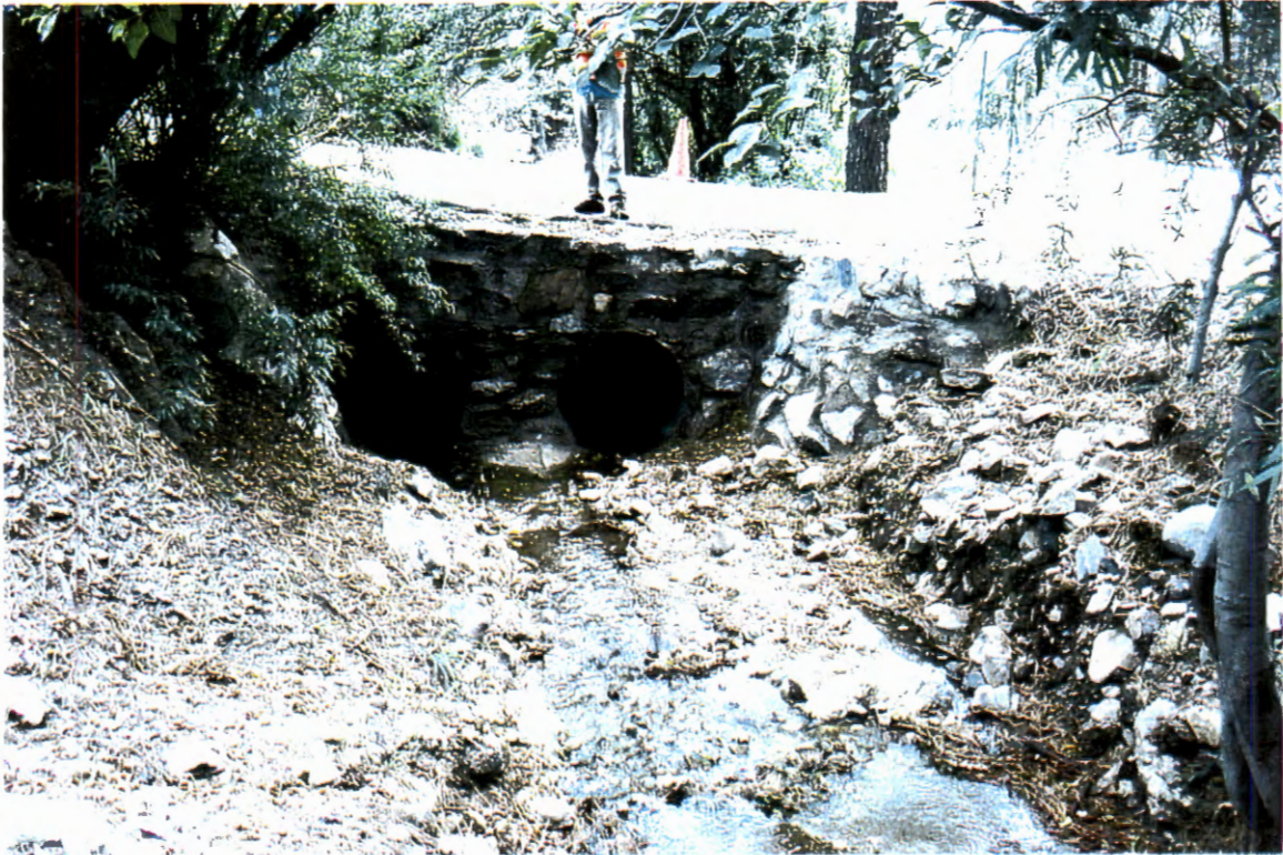
Picture 57. Top of driveway (# 7) looking downstream at 2-36" CMPs (# 6).
