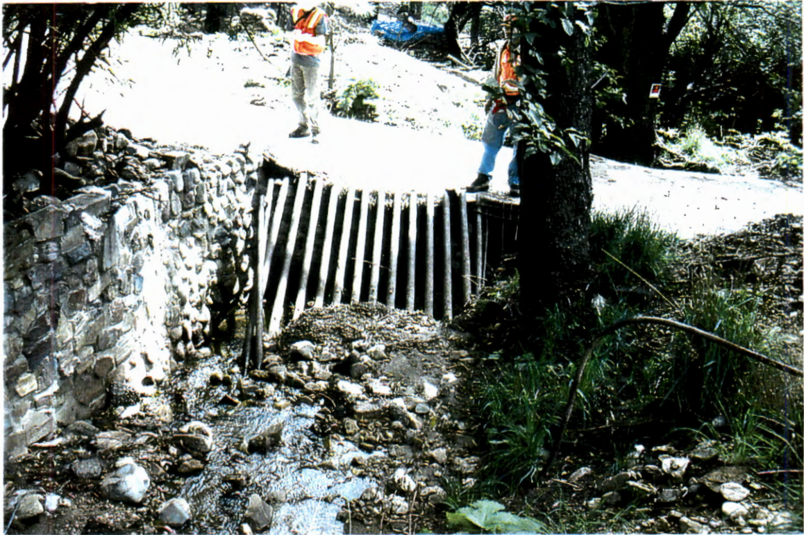
Picture 51. Upstream of driveway culvert (# 5) looking downstream at 2-18" pipes with metal grate.
