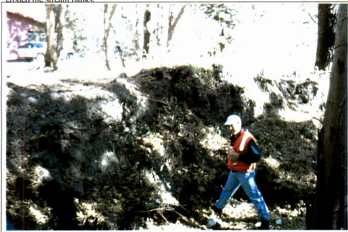
PHOTOGRAPH 123 – Looking downstream from right overbank towards Carter Canyon. Notice the eroded left embankment is six-feet high in this area. The Summerhaven wastewater treatment plant is in the background.
