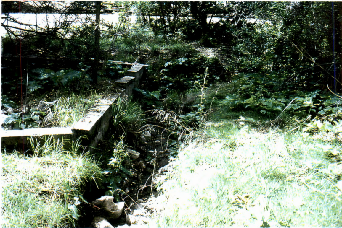
Picture 53. On left embankment looking right at small 2.5' wide and 2' deep channel.
