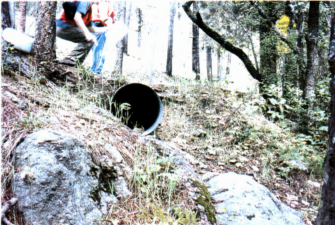
Picture 7. Right side of channel looking upstream at 24" CMP under Sabino Canyon Road.
