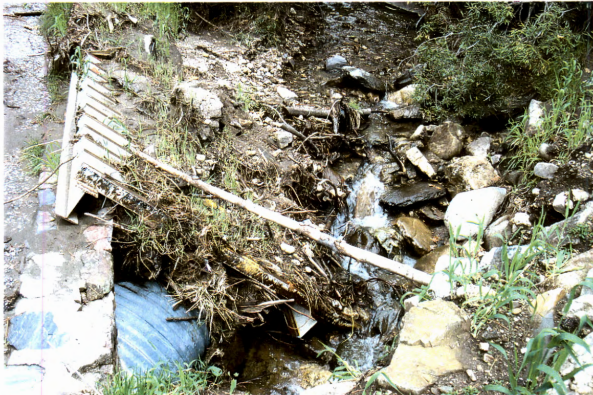
Picture 14. At left side of culvert crossing looking right at grate across culverts (1).
