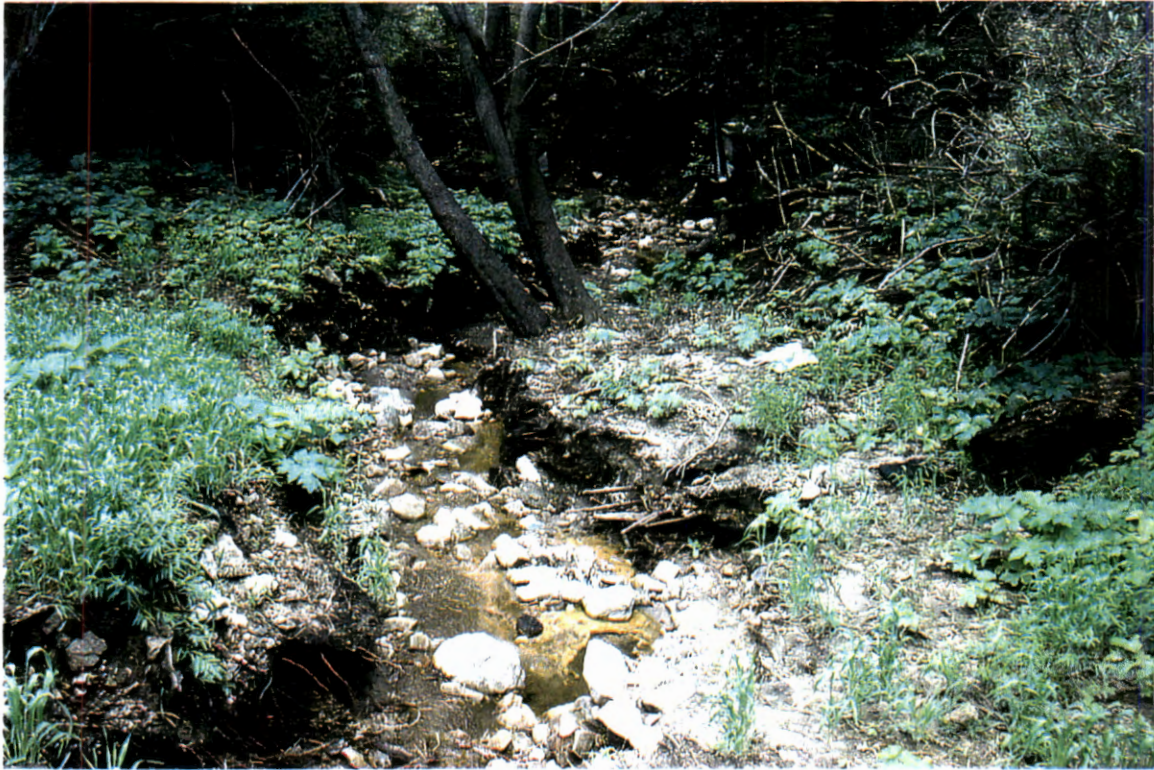
Picture 69. Downstream side of Carter Canyon Road looking downstream at centerline of channel.
