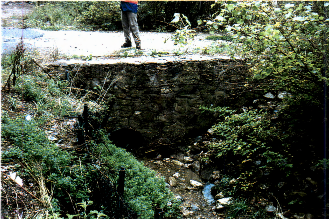
Picture 92. Upstream of driveway culvert looking downstream at 36" CMP and blocked 24" CMP (# 16).
