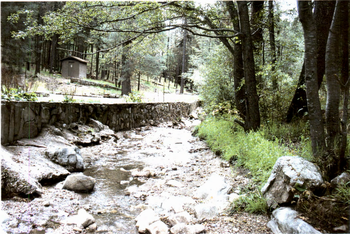
Picture 11. At the downstream side of parking lot culvert (# 1) looking downstream at channel wall on left side.
