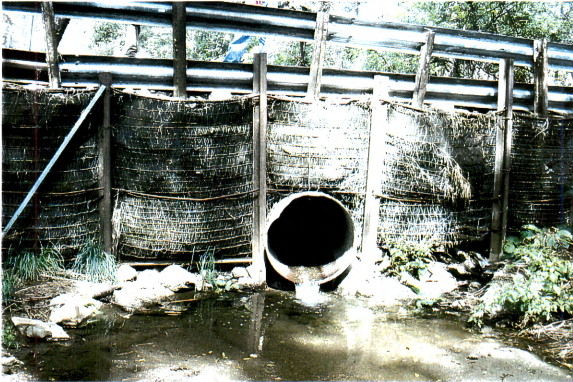
Picture 45. Downstream of Goat Hill Road culvert looking upstream at 3' diameter CMP culvert (# 4).
