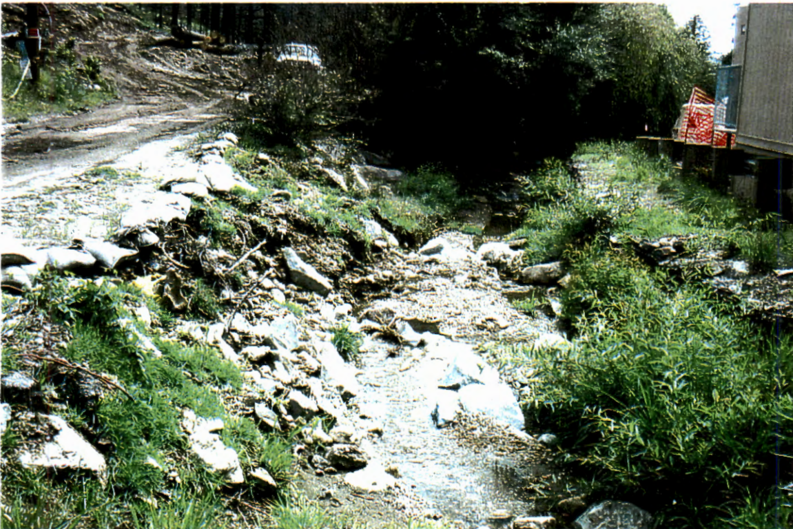
Picture 64. Downstream of Sabino Canyon Road elliptical culvert (# 9) looking downstream at centerline of channel.
