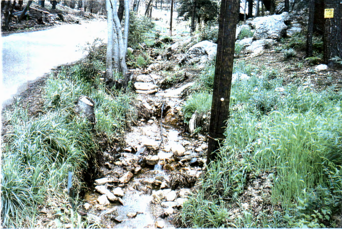
Picture 71. Upstream of Carter Canyon Road culvert looking upstream at centerline of channel.
