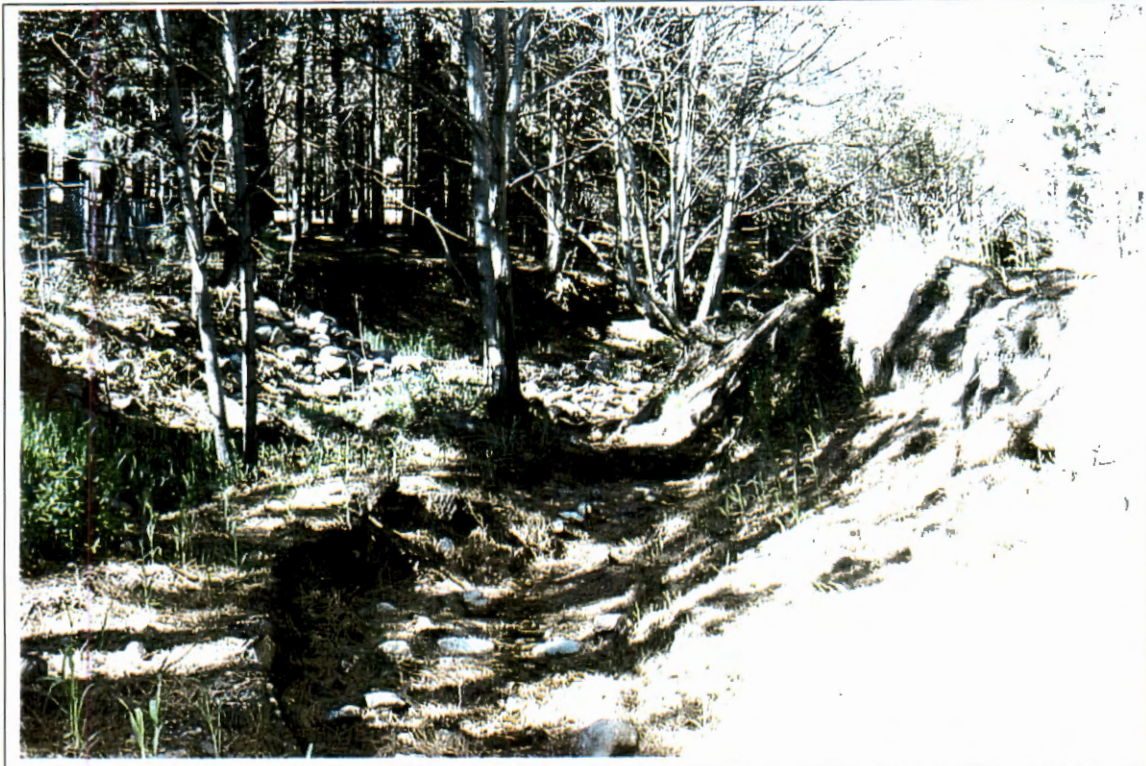
PHOTOGRAPH 122 – Looking upstream at downstream area of Carter Canyon. The Zimmerman Elementary School is at the top of the right overbank area. This is an example of high erosion potential. Revegetation efforts have not succeeded, and high velocity flows have eroded the stream banks.
