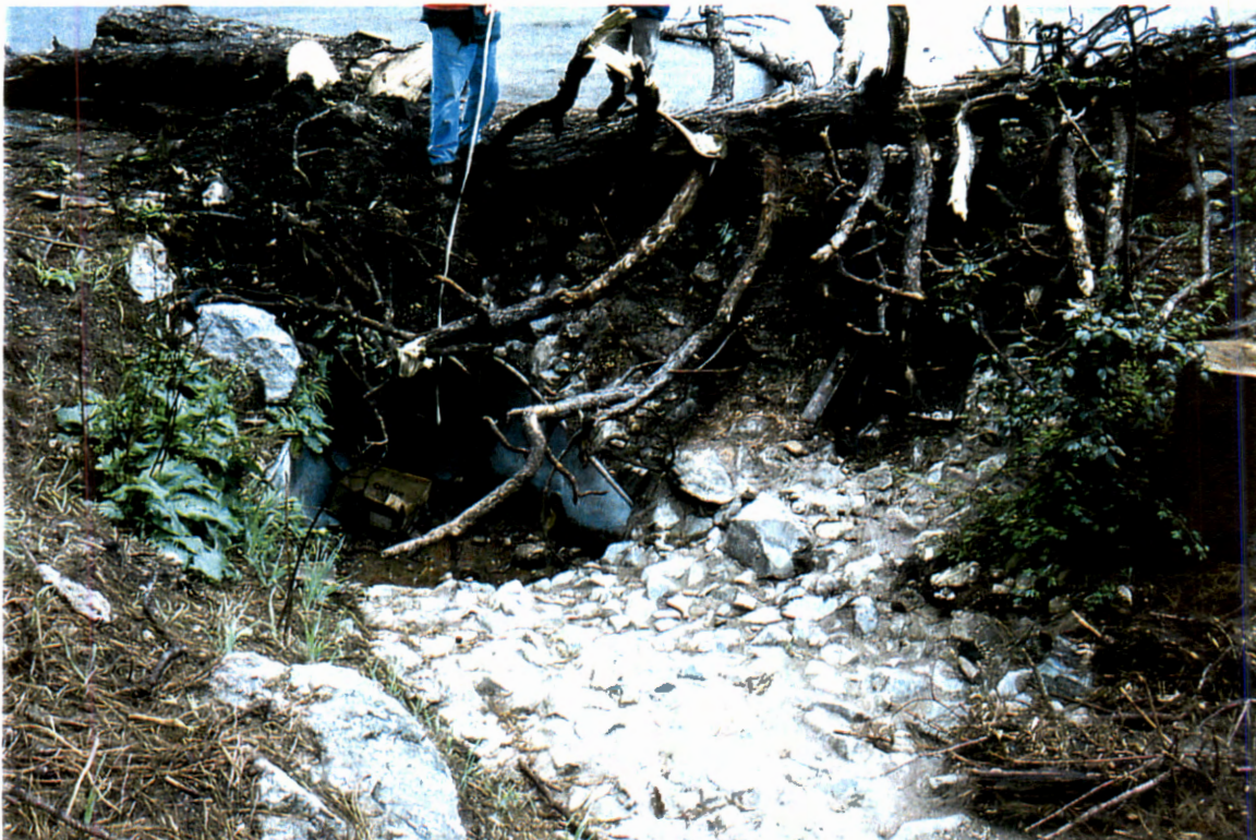
Picture 113. Upstream Tucson Road looking downstream at a 36" CMP (# 21).
