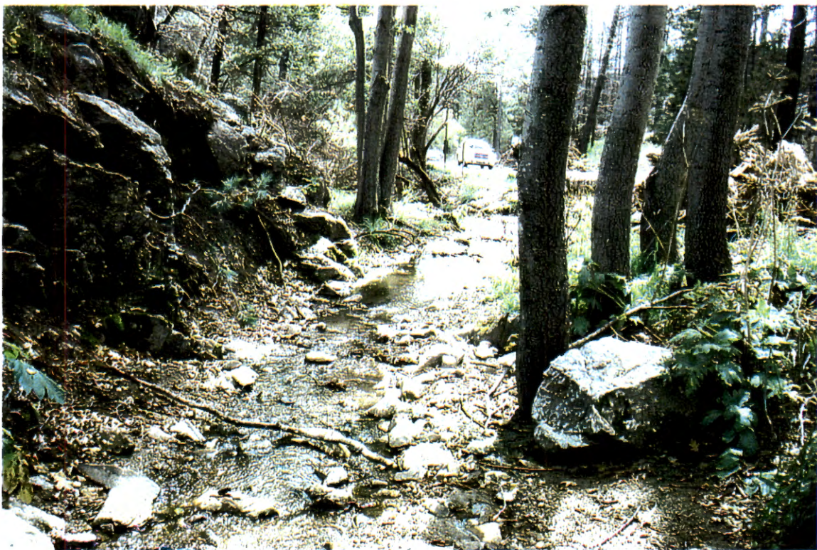
Picture 60. Downstream of coffee house driveway (# 8) looking downstream at centerline of channel.
