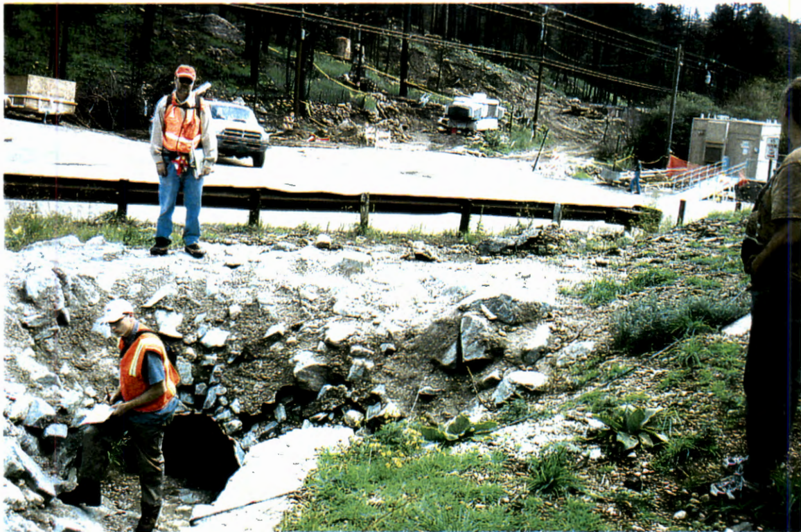
Picture 68. At Sabino Canyon Road looking downstream at culvert (# 9) and Sabino Canyon Road.
