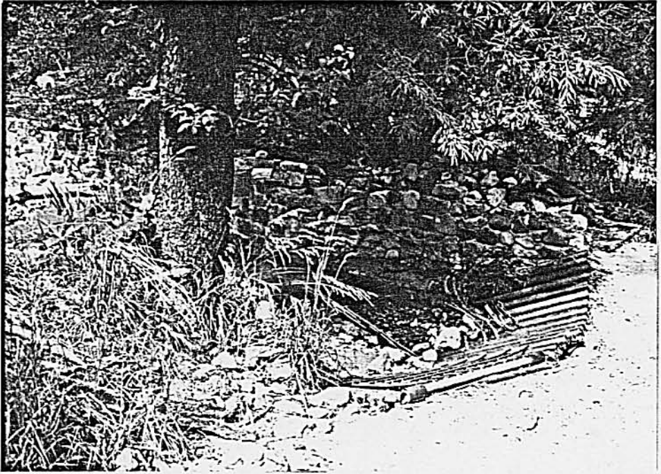
Upstream side of crossing at 12824 Sabino Canyon Park NO PERMIT FOUND
