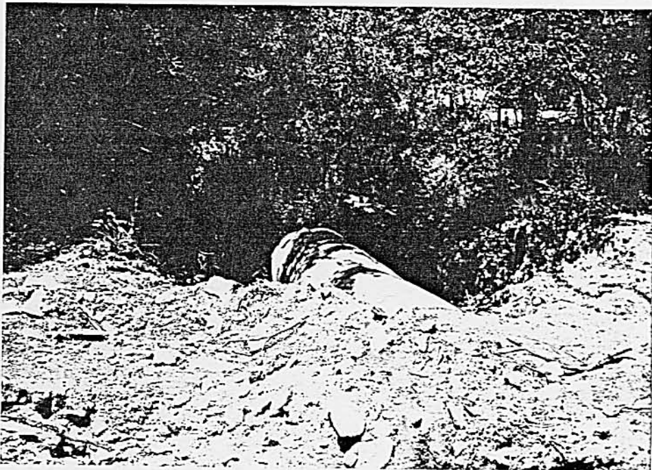
Downstream side of crossing at 11179 Carter Canyon Road. (driveway partially washed out)
