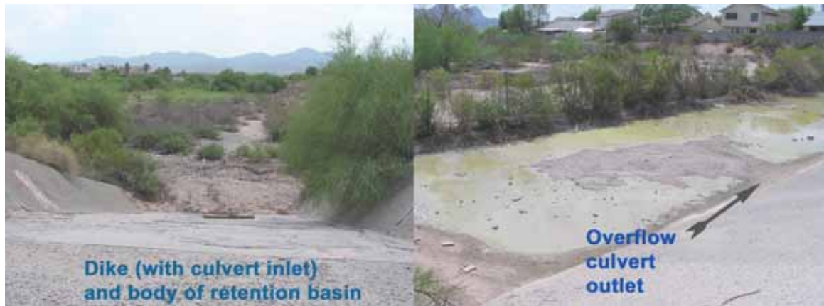
Figure 23. Countryside Detention Basin (Overton Road) in northwest Tucson, with the water detention area and sediment trap (left) with an overflow dike perforated by a culvert leading to a concrete overflow pool that functions as an apron preventing erosion (right). Water detained in the basin flows out through the shallow apron pool, where numerous tadpole shrimp, which eat mosquito larvae, and Couch's spadefoots were found in summer 2006.
