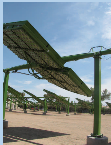
Solar at Drinking Water Facility City of Somerton
