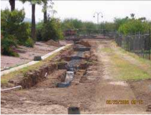
APS Ductbank at TPSS No. 3
