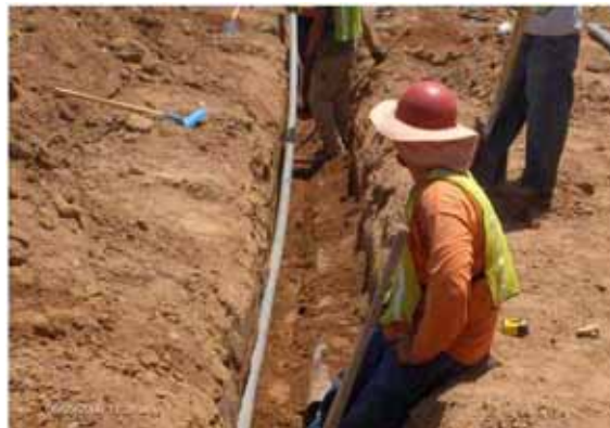
Contractors West using a joint trench to install 2.5- inch and 2-2-inch conduits crossing the LRT 471+30 to the East
