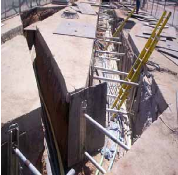
Level 3 relocating manholes on Washington Street from 7 th street to 24 th Street in Line Section 3
