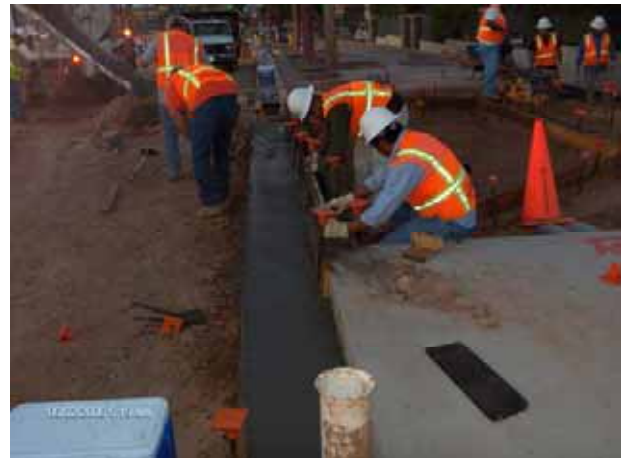
Early morning concrete pour of curb and gutter at Central High School.
