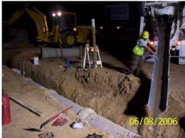
KWC crews placing slurry on the installed storm drain lateral at Sta. 463+80
