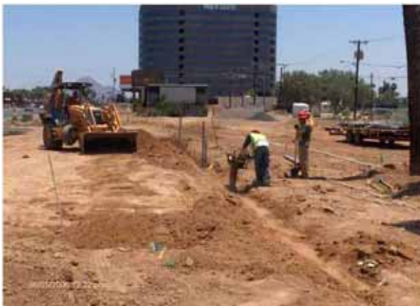
Contractors West compacting the trench backfill crossing the LRT 471+30 to the East
