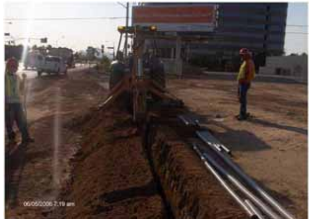
Contractors West excavating the trench for the new 2-inch conduit station 475+64 to 477++ East of Central South of Camelback
