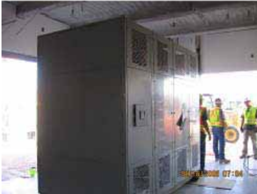
Rectifier Transformer at TPSS No. 9
