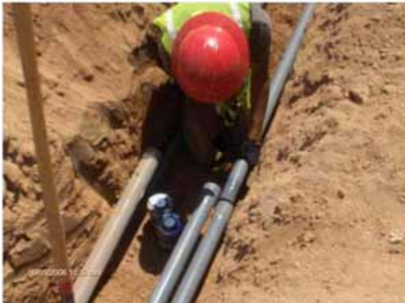
Contractors West installing the new 2-inch conduits crossing the LRT at approximately 471+60
