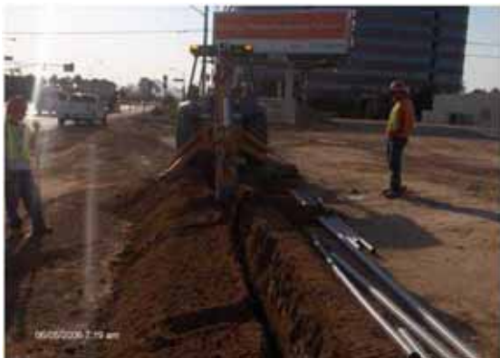
Contractors West excavating the trench for the new 2-inch conduit station 475+64 to 477++ East of Central South of Camelback
