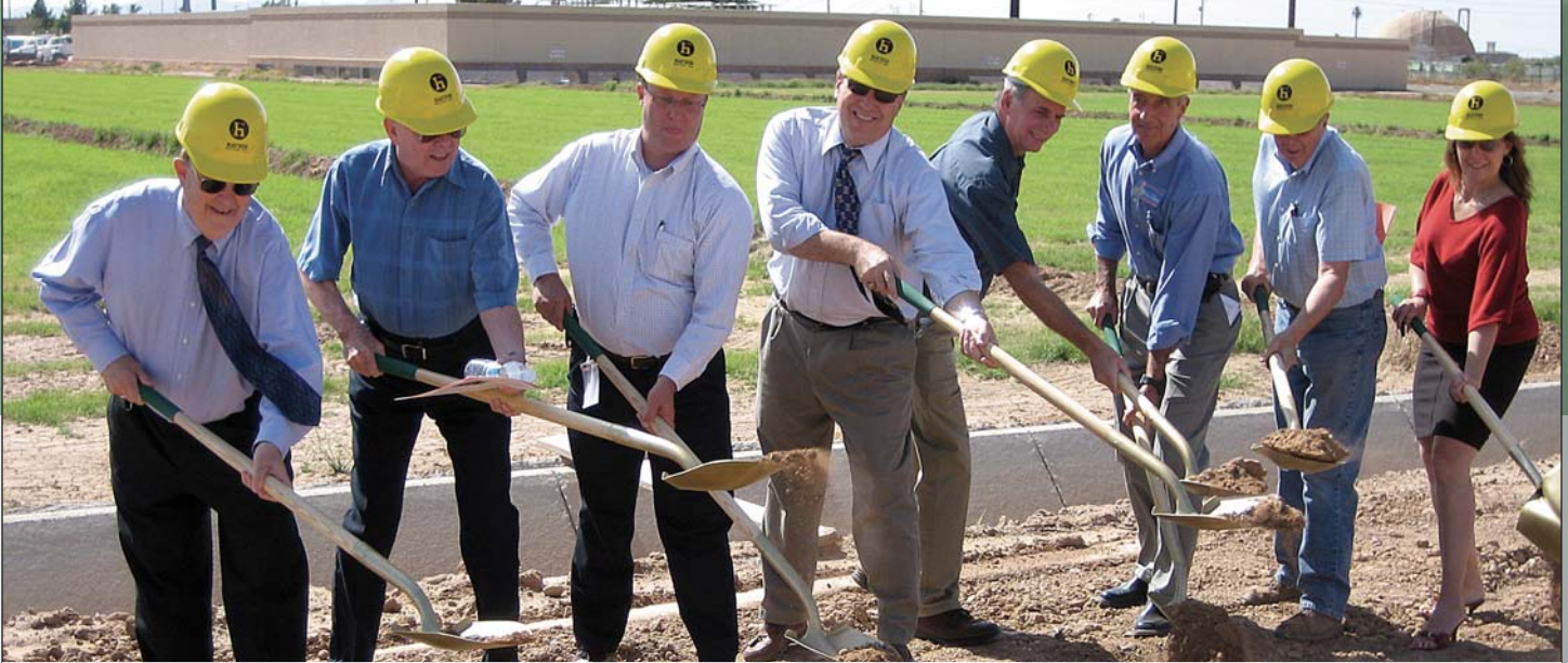
Mayor Dunn invites officials to celebrate the construction of the region's newest park-and-ride.
