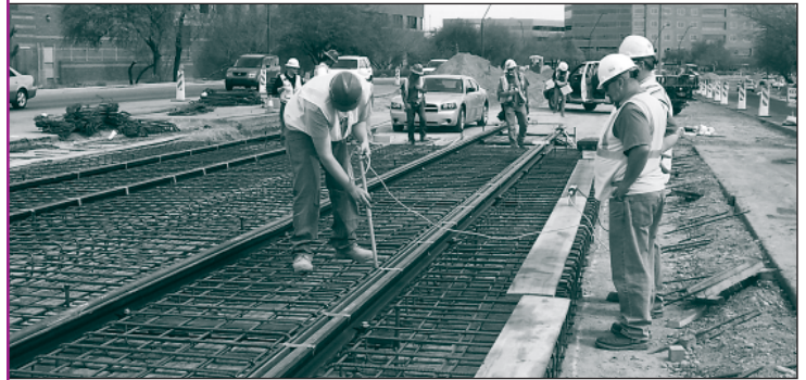
Workers install the first in-street tracks near 56th Street and Washington Street.
