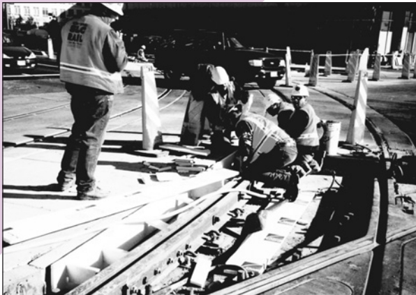
Workers install track on Salt Lake City's Main Street. METRO track construction is slated to begin in February.
