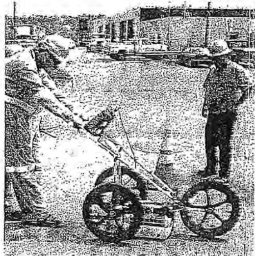
Ground-penetrating radar instrument locates and inspects utilities, part of maintenance quality assurance.
