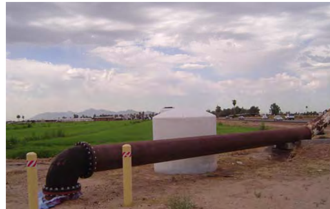
Existing Reclaimed Water Delivery Header
