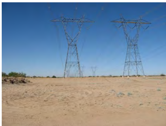
Existing 500kV transmission lines
