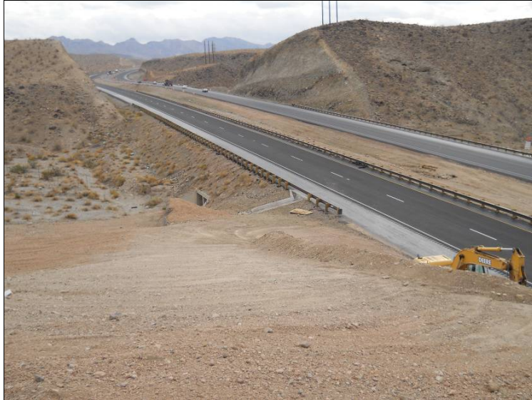
Figure 2. Reconstruction of U.S. 93 (between Mileposts 2.3 and 17) from a Two-lane Highway to Four-lane Divided Highway.
