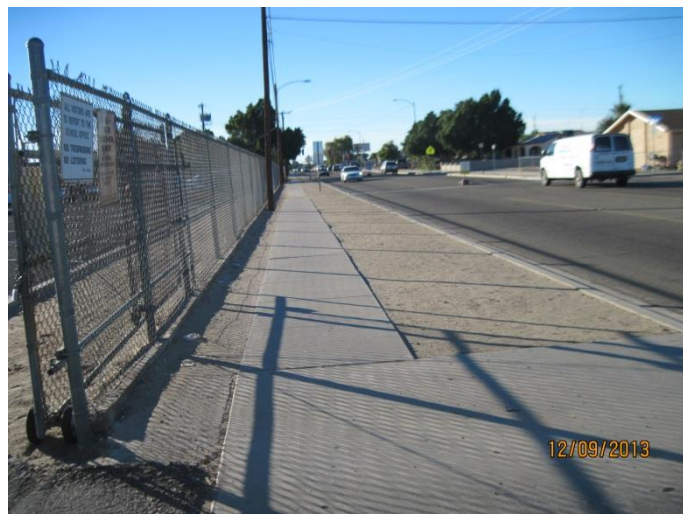
Detached sidewalk along east side of Arizona Avenue in front of school
