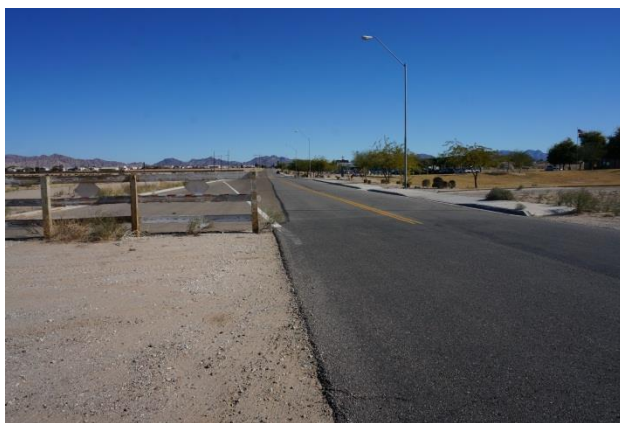
Scalloped roadway on 28th Street, west of school
