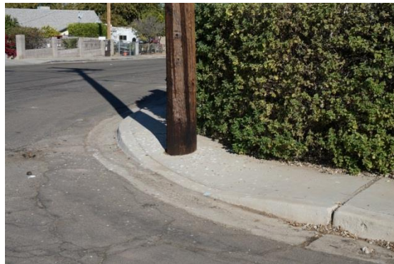
Utility pole obstructing sidewalk accessibility
