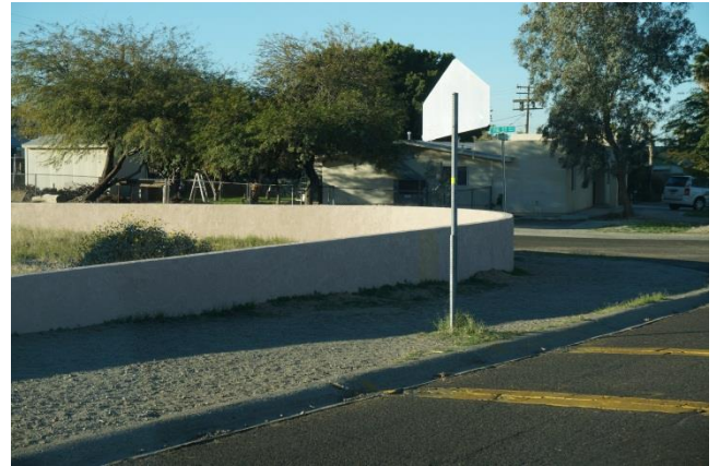
Lack of accessible ramp at mid-block crosswalk on Park Lane
